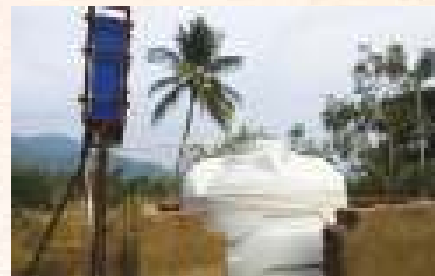
Installation of gravity flow based ultra-filter-Rachuli village, Harsha Trust
