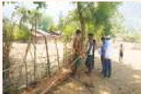
Pipe line demarcation and measurement at DBI site of Partner NGO-COFA, Odisha
