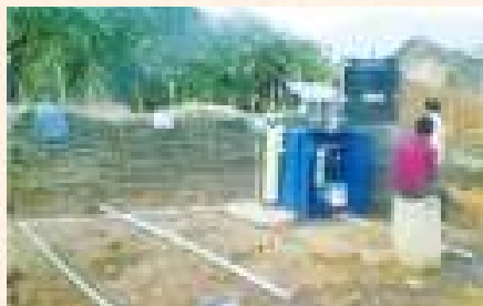
Installation of Gravity flow Micron & Carbon filter with solar based UV -Duruguda village, Harsha Trust
